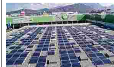
Riesige SEP-Photovoltaikanlage (SEP)
